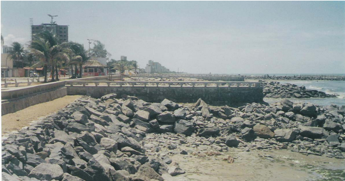
Figure 4 - Edge of Olinda, “Senator Marcos Freire” Avenue, where if they can notice the workmanships of containment of the advance of the sea where long ago the Bar’s existed that had been transferred to the left side of the avenue.
